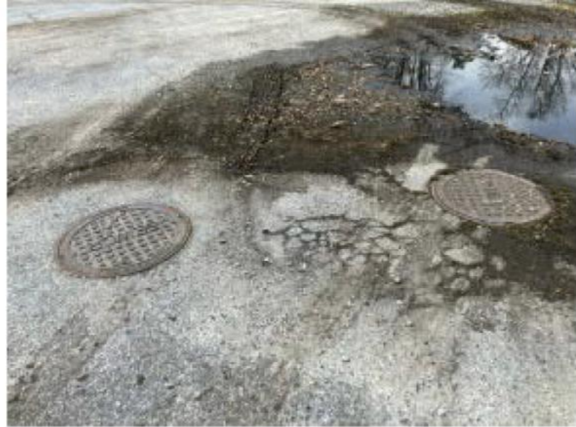
Photo #2 View of the grease traps behind Glenda's.
